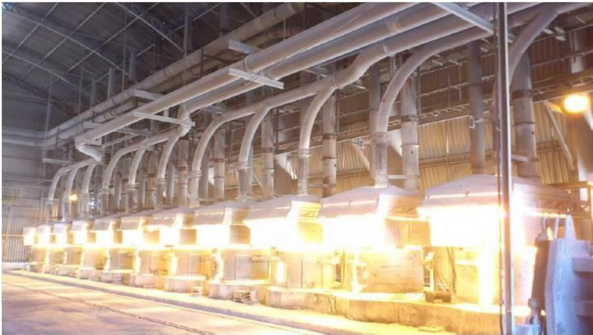
Figure 9: Battery of zinc oxide production furnaces
